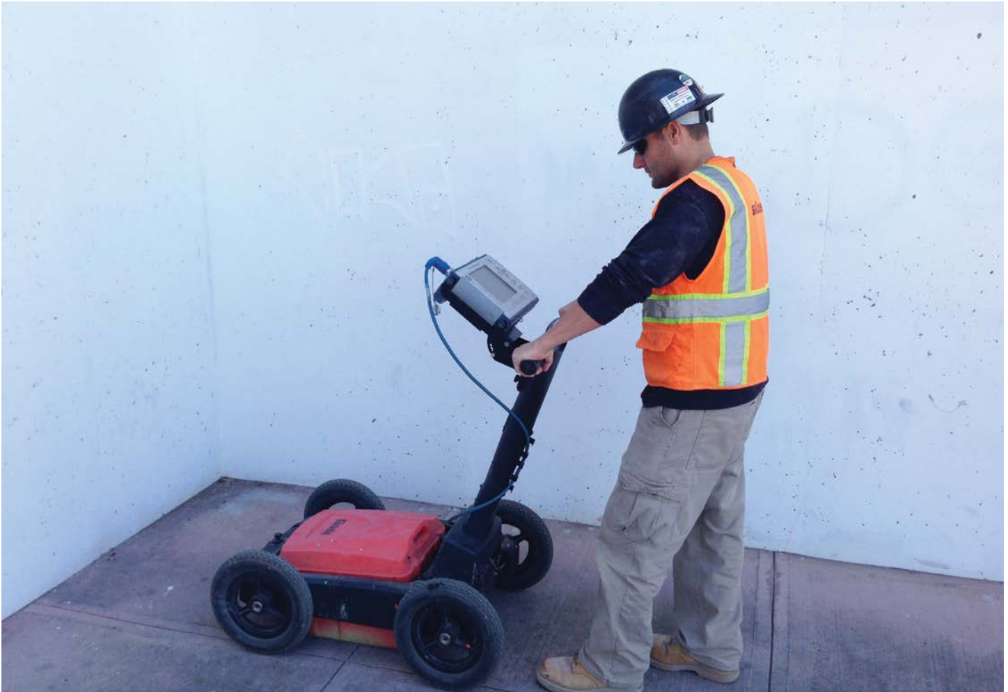
A 400-MHz antenna was used to locate and identify utilities buried up to 5 feet deep in reinforced concrete.
