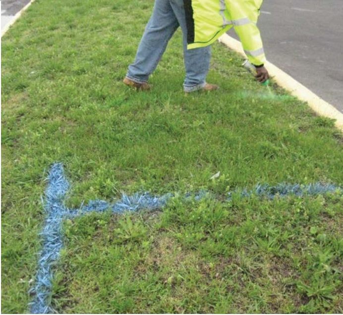
All electrical, gas, telephone, sewer and water lines were identified with APWA uniform color codes.
