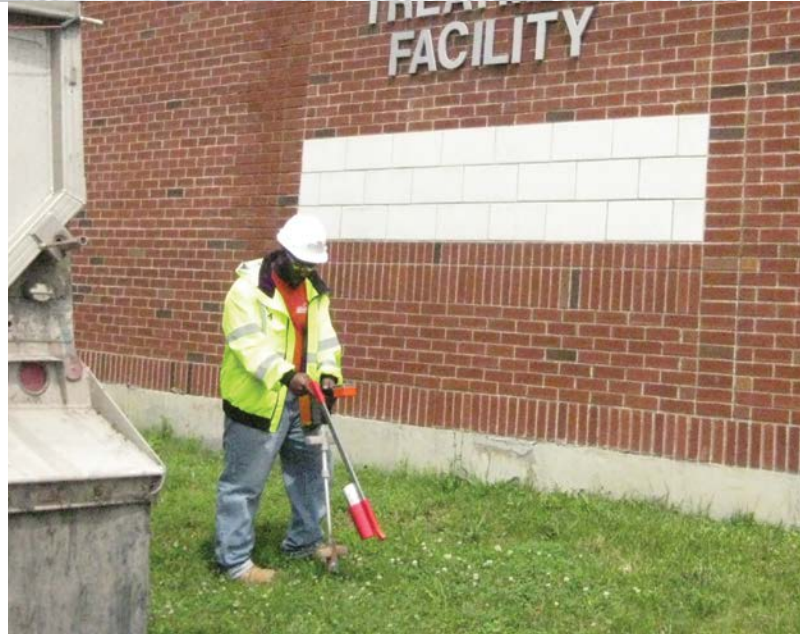
The results have helped engineers with the design of a new sewer system.
