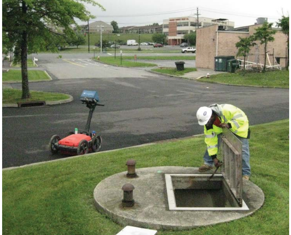
The equipment was used to cover an average of 460 feet per hour.
